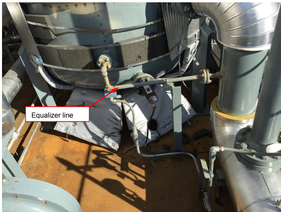
Figure 2. Equalizer line between the discharge line and oil separator vessel
