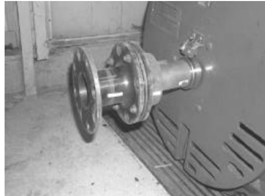
Figure 2. Coupling on 600 HP motor
