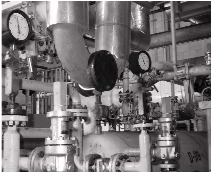
Figure 2: Discharge piping from vessel D118 with de-tuning weights secured.
