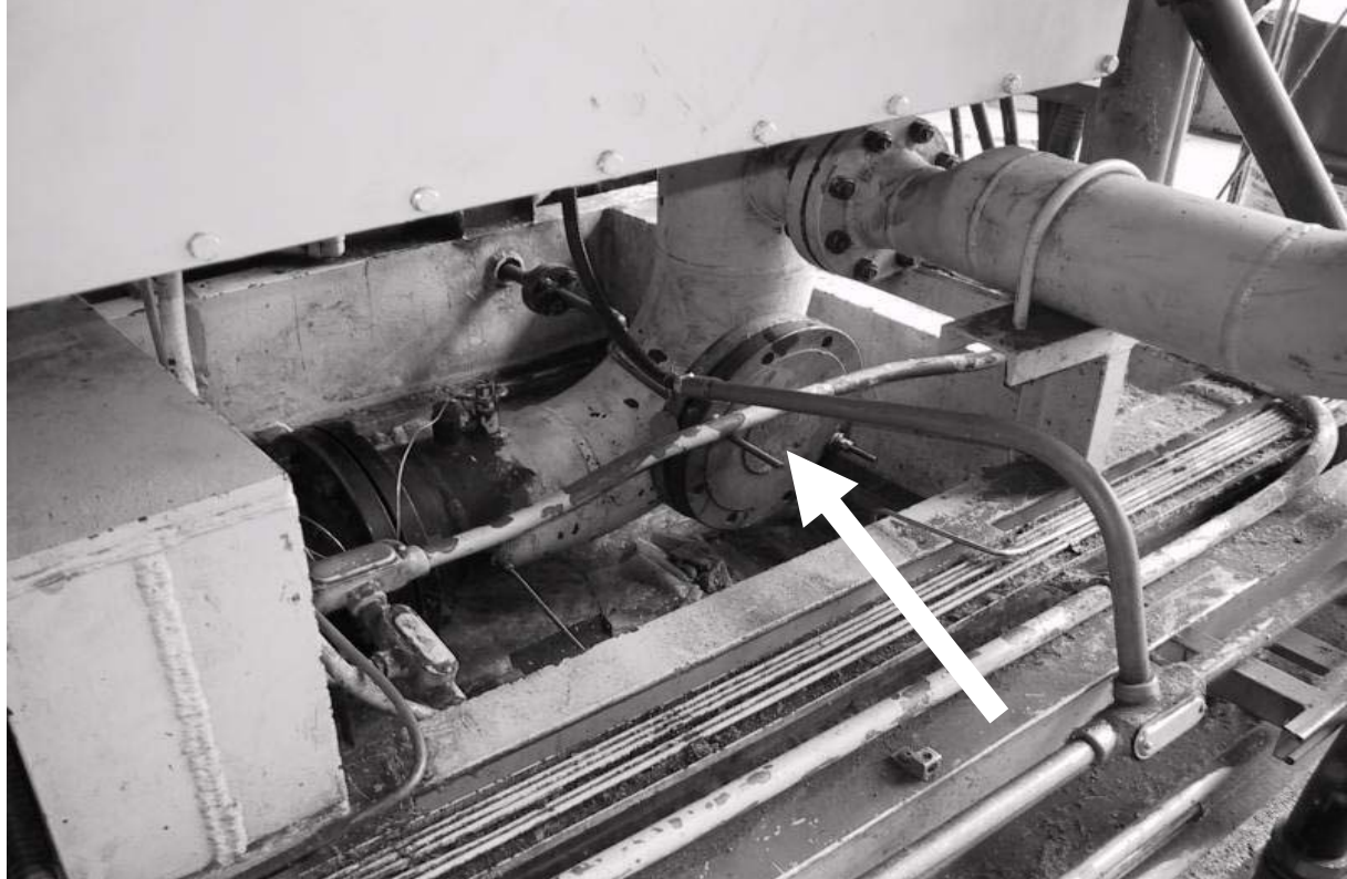
Figure 5: Discharge line de-tuning weight located at lower elbow before D118.
