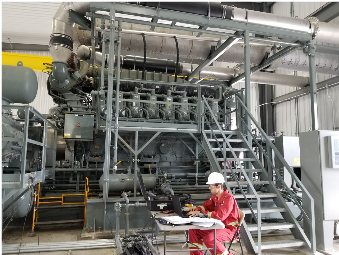
Figure 3: Photo of engine and compressor package – right side
