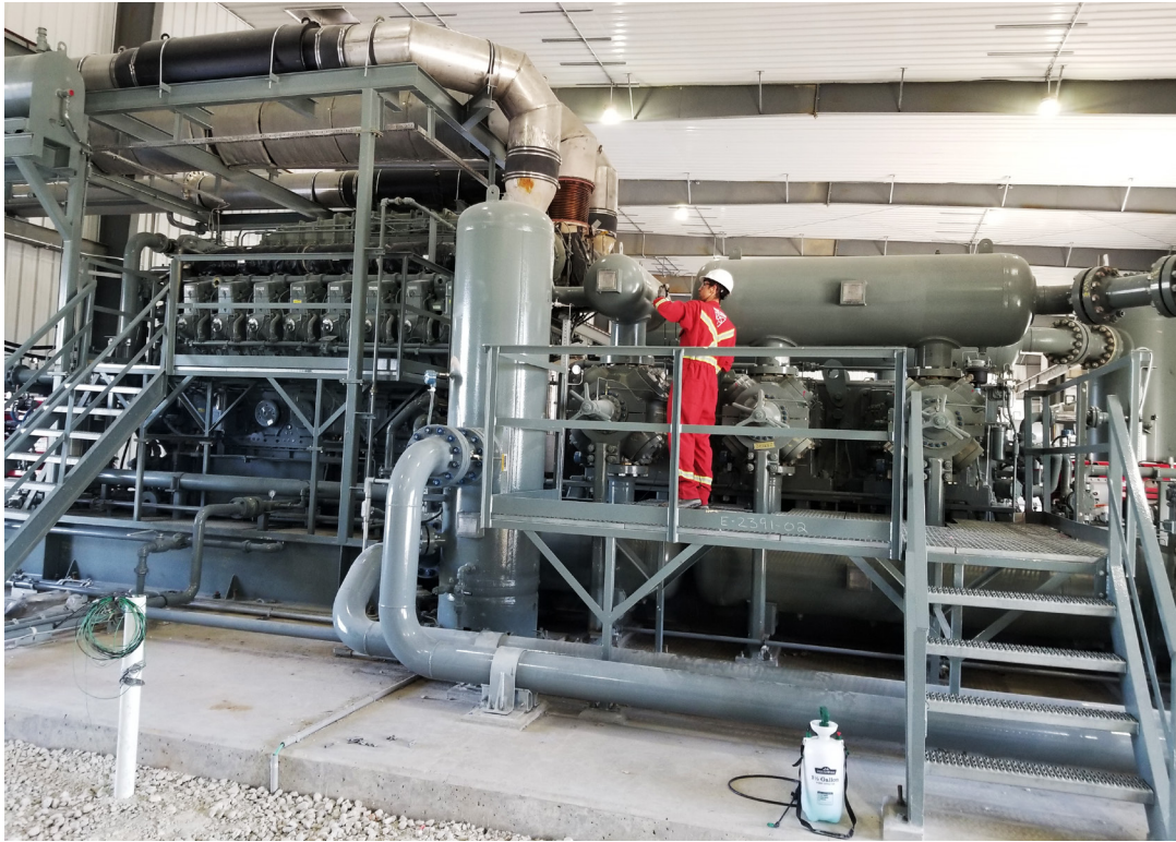
Figure 2: Photo of engine and compressor package – left side
