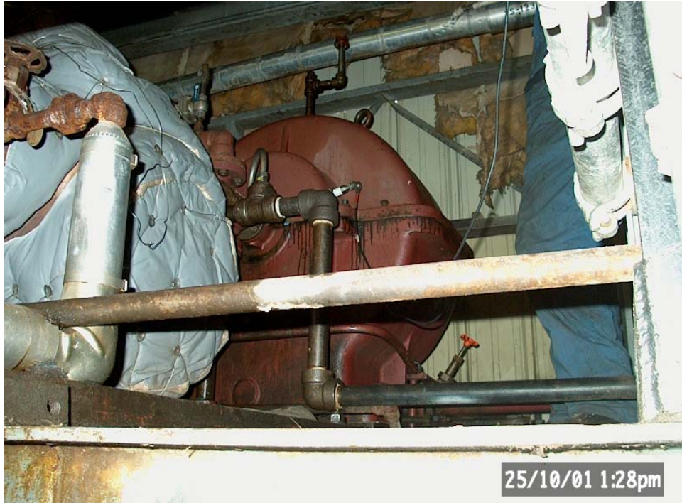
Picture 2: View of Test Point 5 with accelerometer mounted with stud on nut glued to box in Horizontal orientation. The oil pump is on the turbine side of the low speed shaft.
