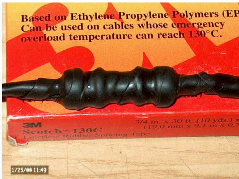
Figure 6. A BNC to BNC connection covered with electrical splicing tape to make water resistant.
