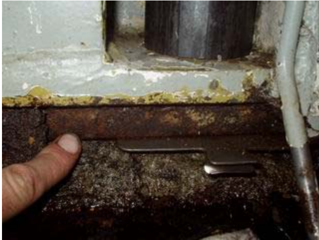
Figure 5: Photo of actual grout connection. Finger points to shimming location between rail and top of grout.
